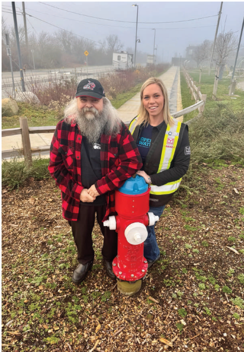
Darcy and Rick with a Clow iHydrant, monitoring Tsawwassen First Nation's water distribution system pressure and temperature.
