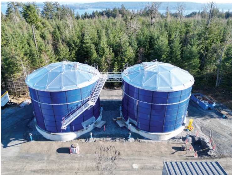
New 1,000 m 3 Water Reservoirs
