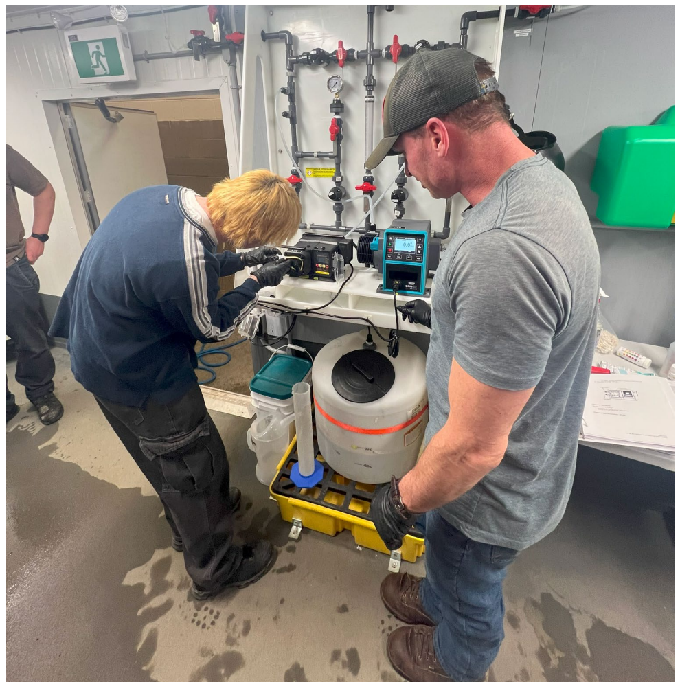
Alex (Engineering student) and Aaron (Operator) doing maintenance work on the sodium hypochlorite pump
