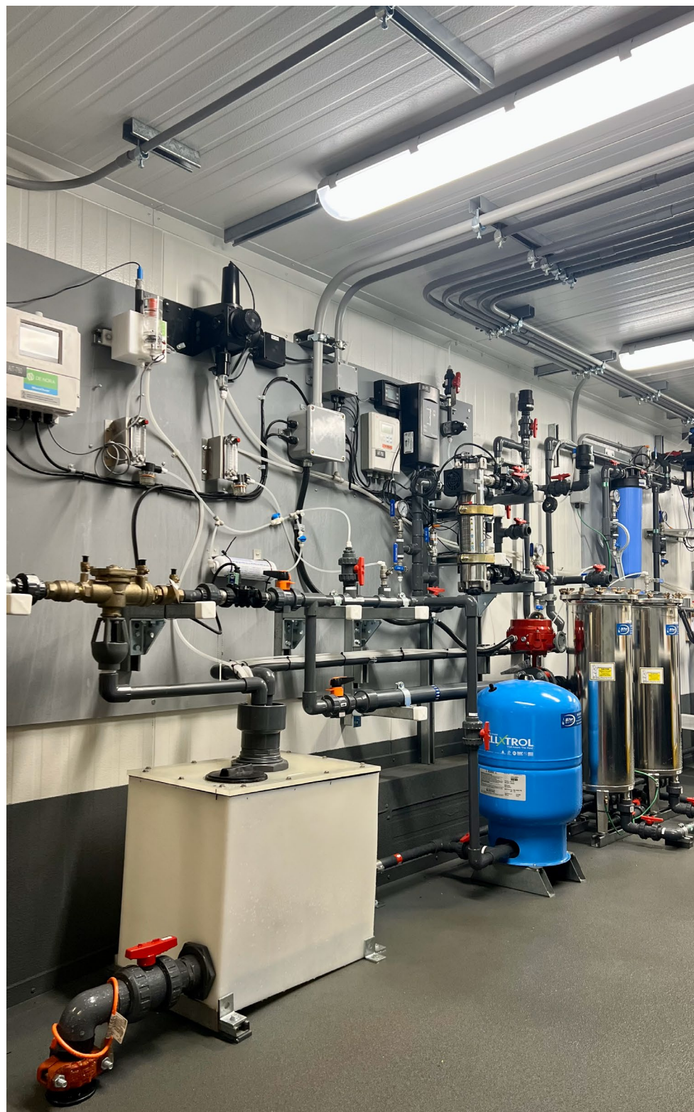
Interior view of Yukon University's Mobile Water Treatment Plant
