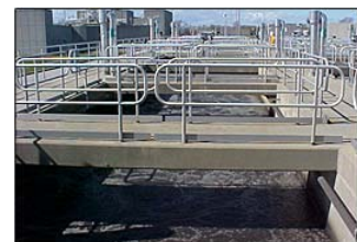
Solids Contact Tanks
