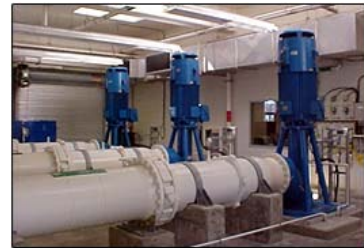
Tricking Filter Pumps
