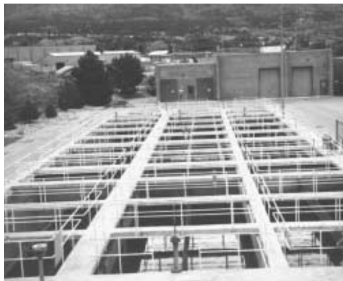
Chlorine & Sulfur Dioxide tankage with degrit and (headworks) bar screen bldg in the background.
