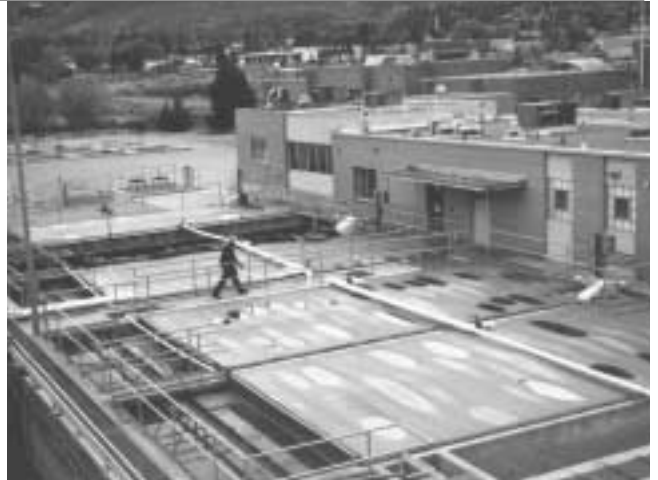
Primary tanks with odor covers & odor line.
