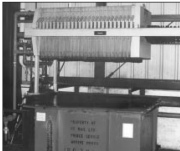
Hydraulic Sludge Press
