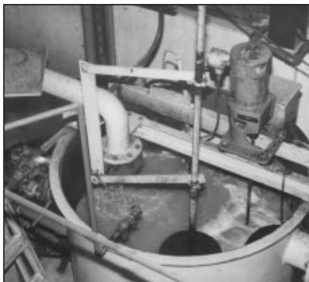
Flocculation Mixing Tank
